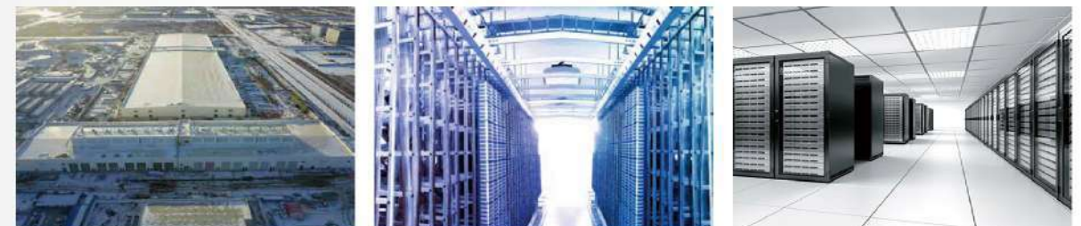
Cloud Data Center
